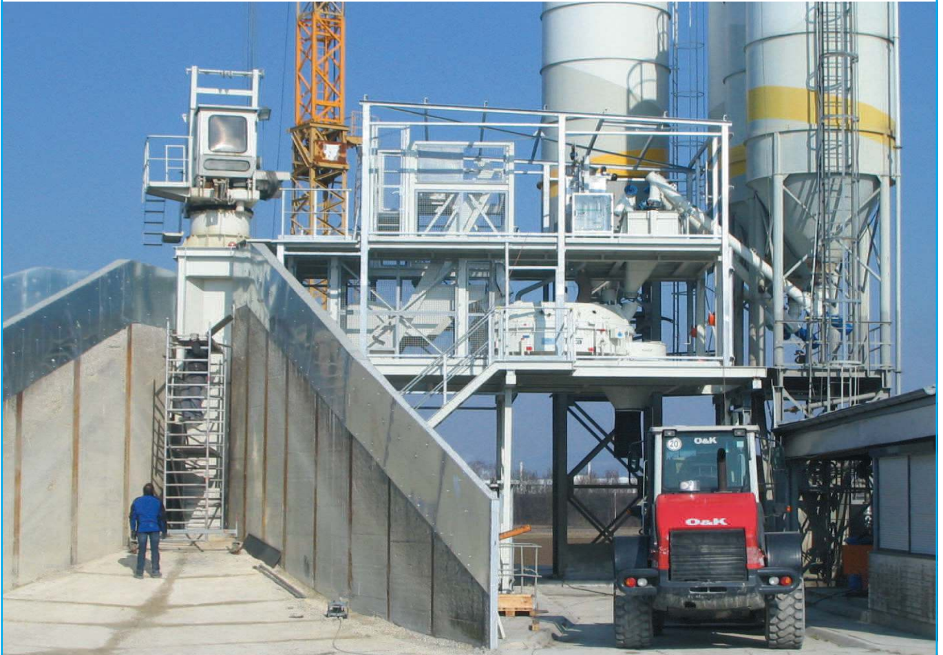
Montage MIXOMAT THZ 3000 B - S 6 Sternanlage • Erection MIXOMAT THZ 3000 B - S 6 scraper system
