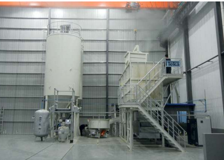
In-line silos and cement silos
