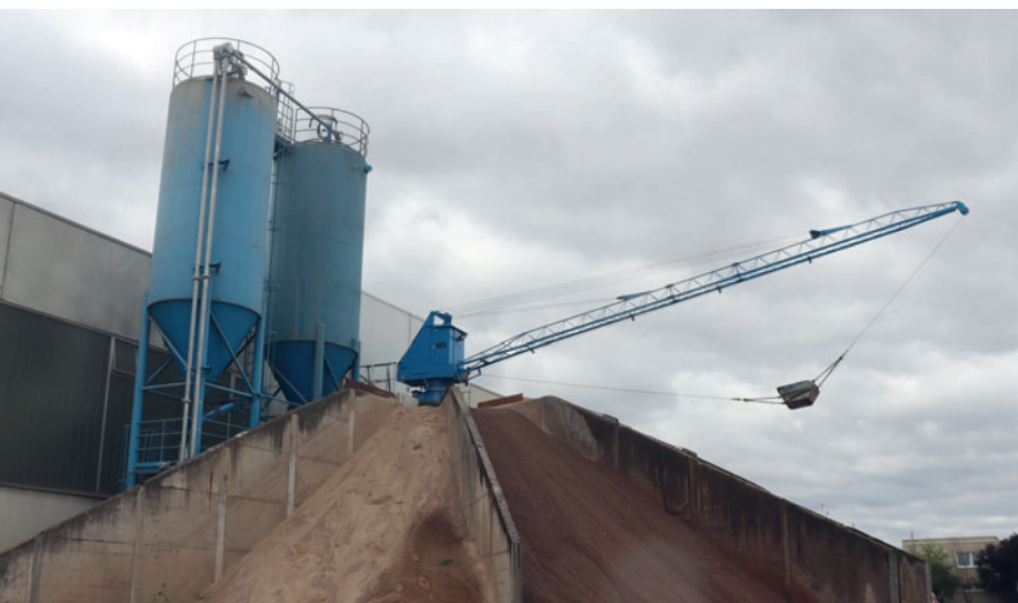
As part of the modernisation, the Arnstadt site was also equipped with a powerful Teka THS 15 automatic scraper.
